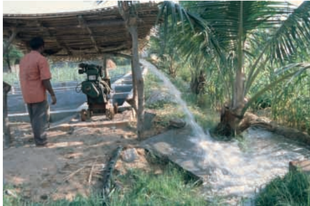
Pilot plant near Madras (Chennai), India. After Treatment in an ÖKOTEC plant the waste water of a boarding school is used for irrigation of paddy fields.
