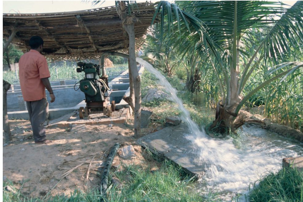
Pilot plant near Madras (Chennai), India. After Treatment in an ÖKOTEC plant the waste water of a boarding school is used for irrigation of paddy fields.
